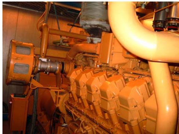
Pic. 1: Caterpillar engine 760 kW power
