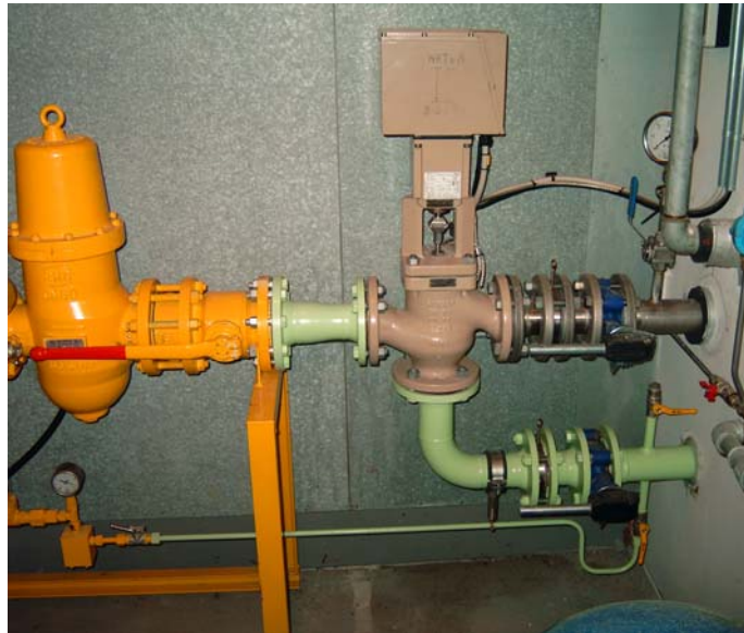
Pic. 2: 3-way valve for fully mixing natural gas and biogas rig
